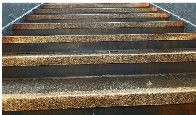
The mud on the painted edging of the steps - before
